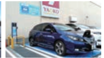
EV charging stations
