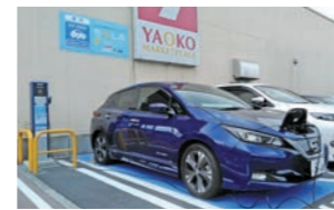
EV charging stations
